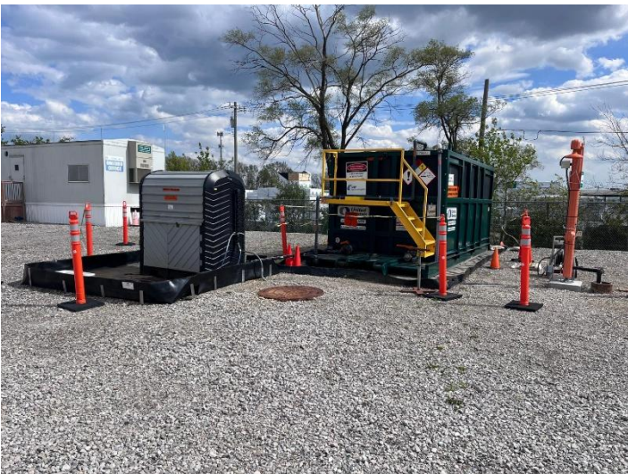
Ferric chloride temporary pumping station at PCI-4-MH-106
