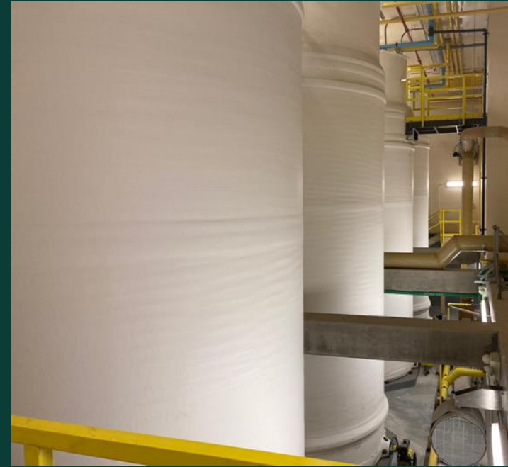
150,000 gallons sodium hypochlorite storage
