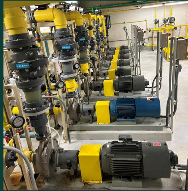
8 chemical feed pumps
