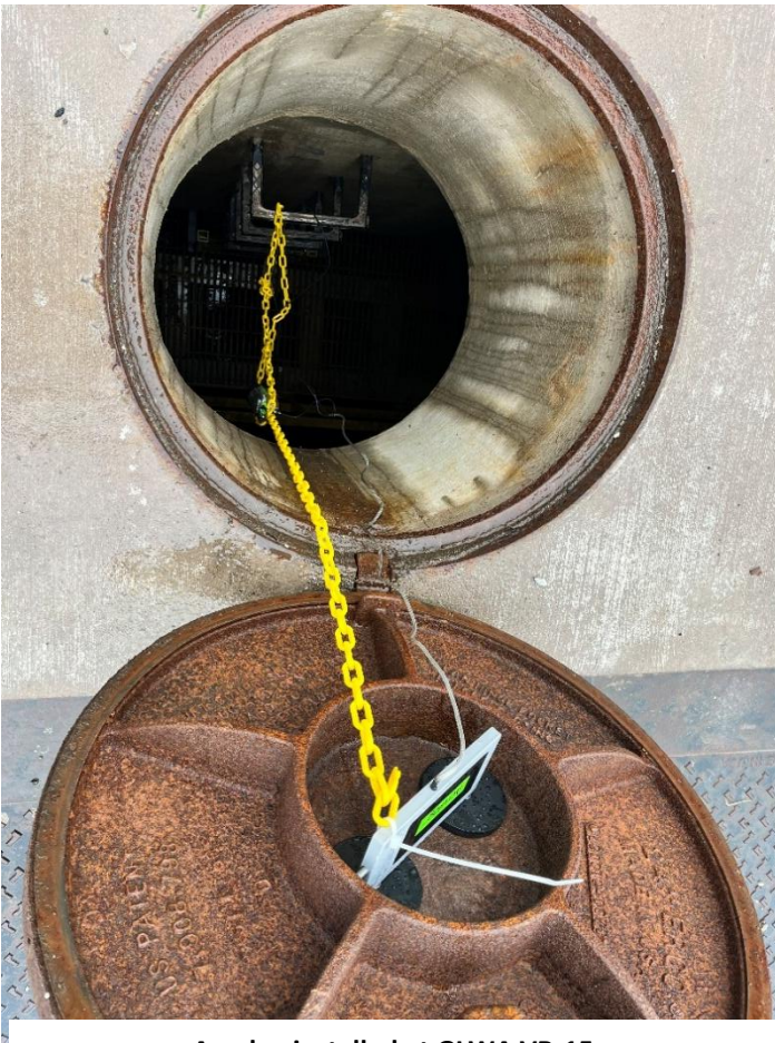
Acrolog installed at GLWA VR-15
