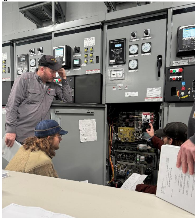
Preventative maintenance and troubleshooting of Sanitary Pump #5
