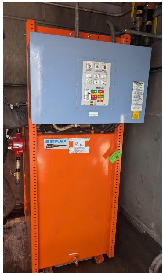
Newly installed day tank for standby generator
