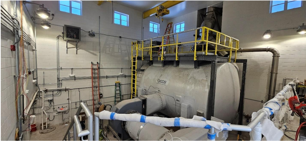
Carbon vessel and blower in ST-S-3 site replica house (looking southeast)
