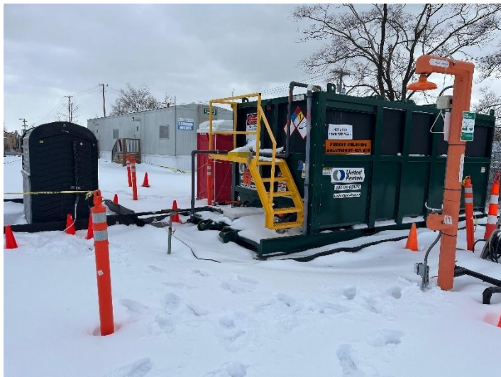
Ferric chloride temporary pumping station
