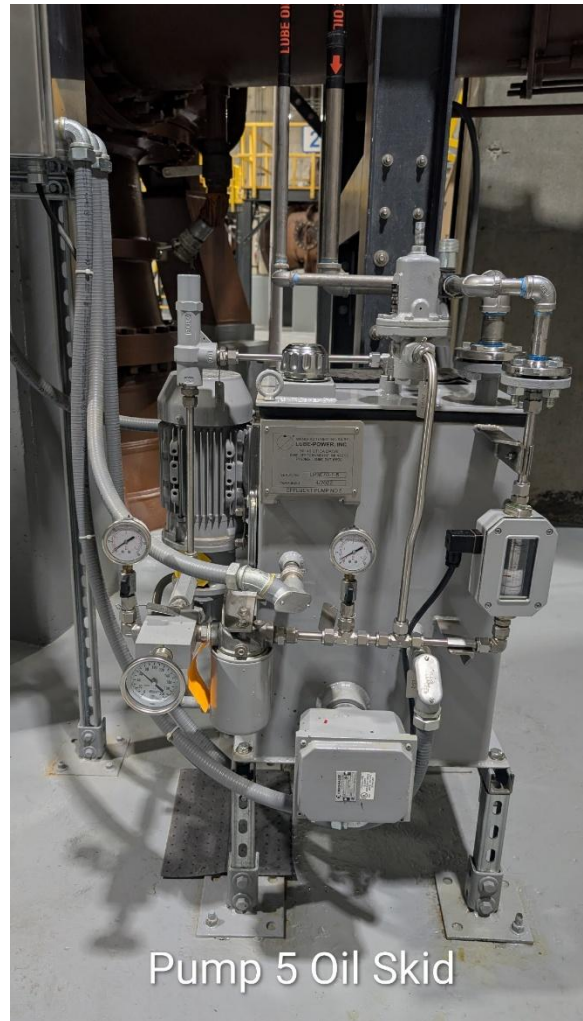
Pump #5 oil skid
