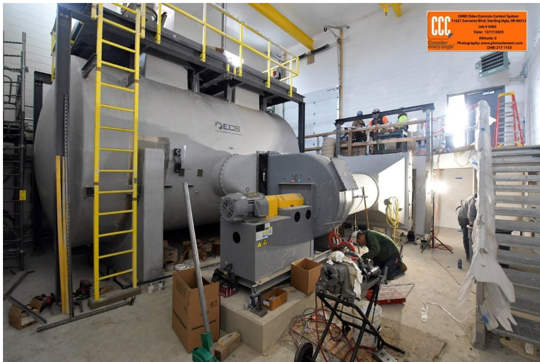
Carbon Vessel and Fan in Replica House (looking southeast)
