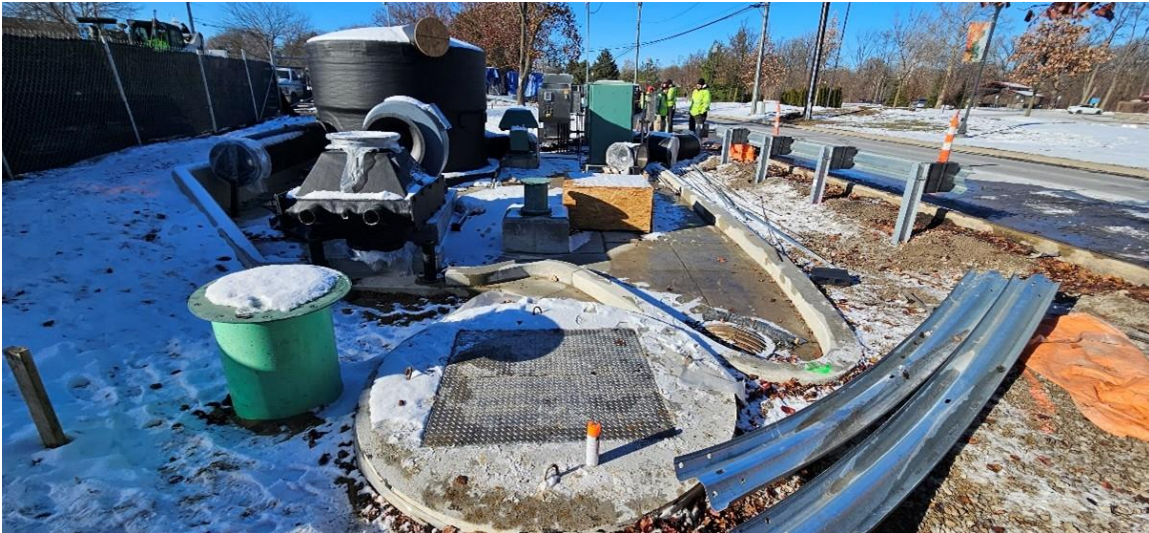
ST-S-1 site construction status (Dodge Park Road and Utica Road, looking east)
