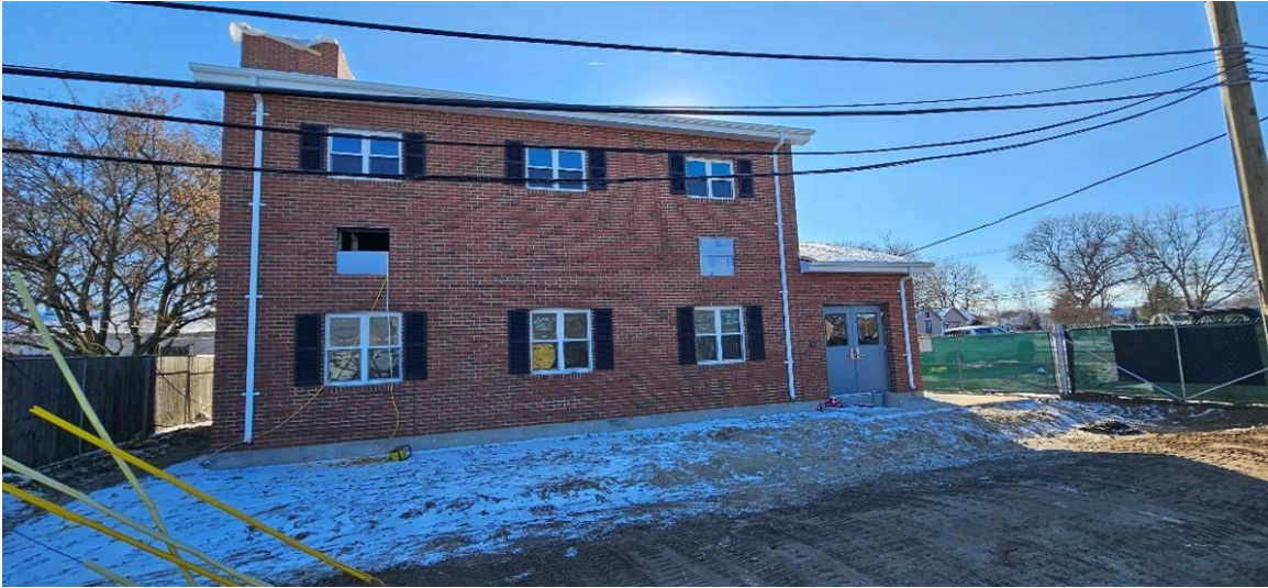
Construction of brick face of north wall at ST-S-3 site (looking south)
