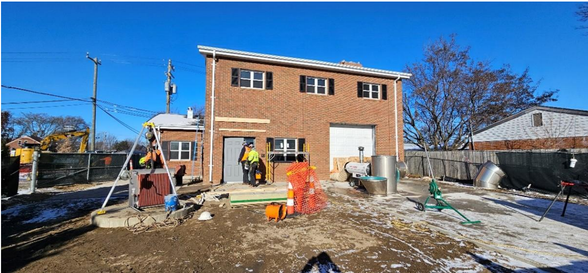
Construction of brick face of south wall at ST-S-3 site (looking north)
