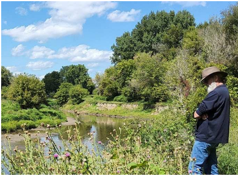
Inspect ID: 2025-10019 Rated Item: 4. Erosion Lat/Long: 42.53211/-83.01538 Caption: 10019 - Erosion along riverbank.
