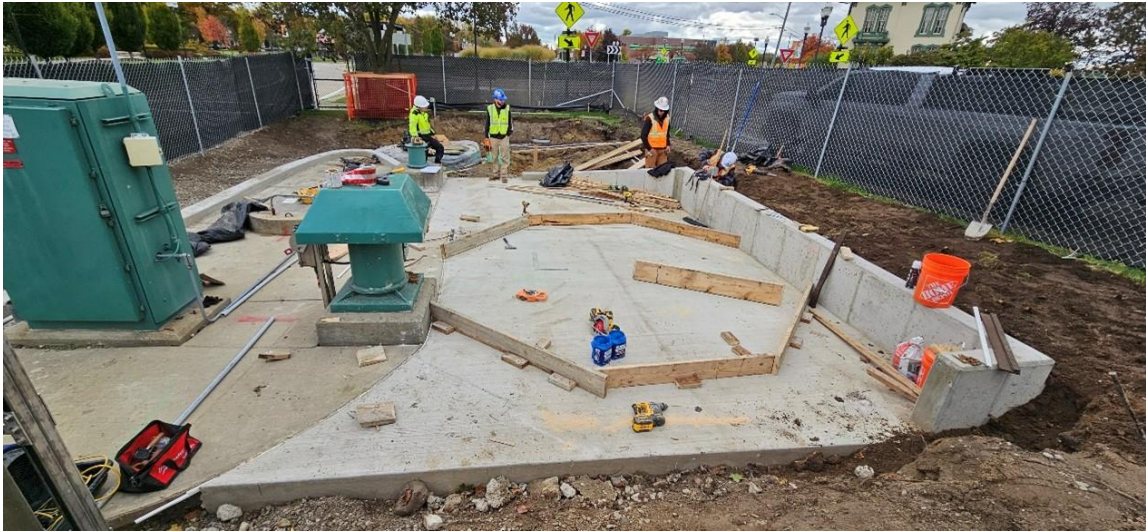
ST-S-1 site construction status before vessel pad construction (Dodge Park Road and Utica Road, looking east)
