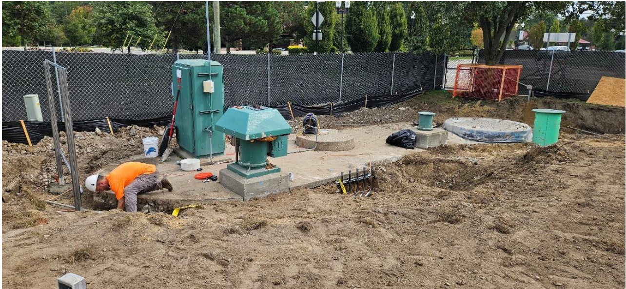
ST-S-1 site construction status (Dodge Park Road and Utica Road (looking northeast))
