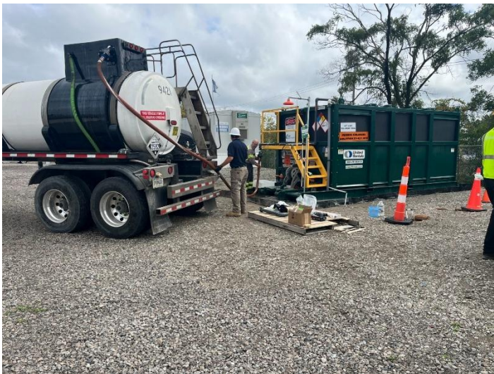
Ferric chloride delivery at NESPS
