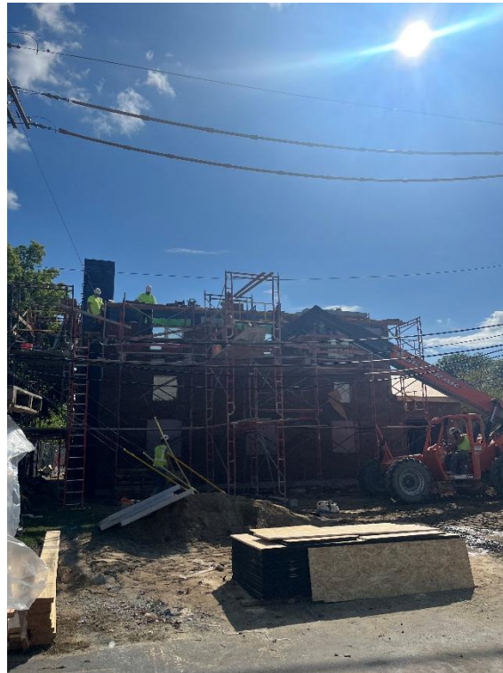
Construction of brick face of north wall at ST-S-3 site (looking south)
