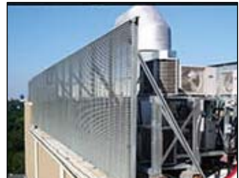
Visual Screening of HVAC System
