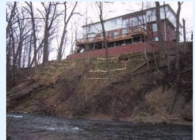
This home is threatened by bank erosion along the Clinton River in Rochester Hills.
