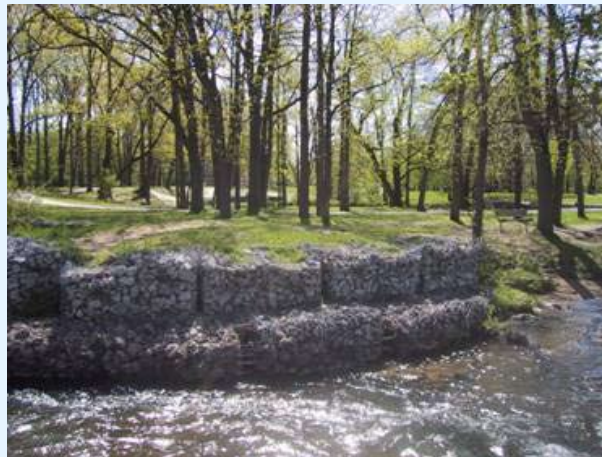
The banks of the Paint Creek in the City of Rochester Municipal Park are stabilized by gabion baskets.
