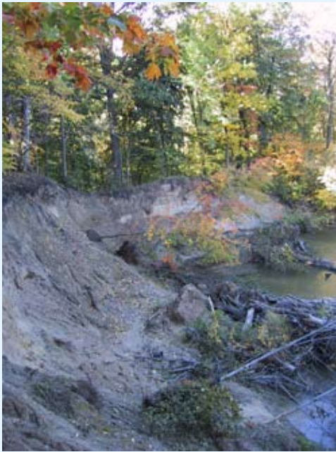
The riparian forest is falling into the river as the Clinton River erodes its banks.
