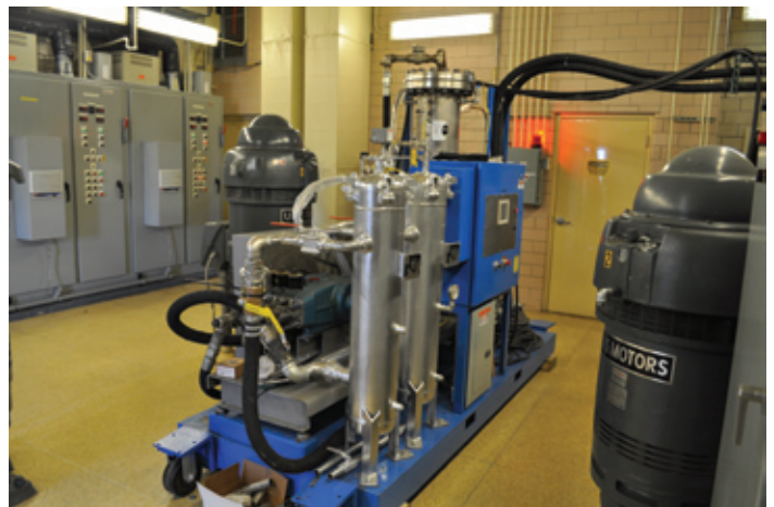
DynamOx, a Michigan based start-up manufacturing company, is working with H 2 O opportunities to demonstrate the effectiveness of supersaturated oxygen as a “green solution” in eliminating corrosion in sewer systems thereby extending system life and protecting the health and safety of workers and residents.
